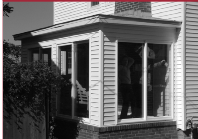
Volunteers help put the finishing touches on TWC’s new all seasons room in Kent County.
